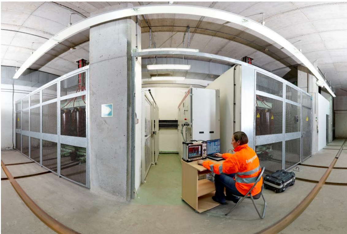
Figure5. Photo of the system installed on the substation.
