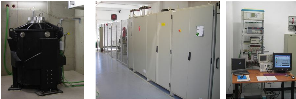
Figure 6. Machine and Flywheel installed in the substation, power electronics converters and control
